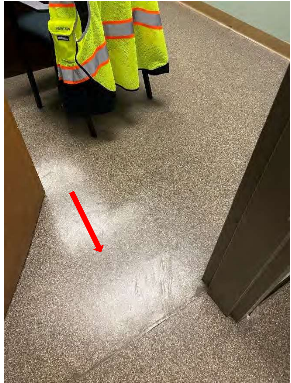
The gray sheet vinyl flooring and the yellow mastic used to attach it are asbestos-containing.
