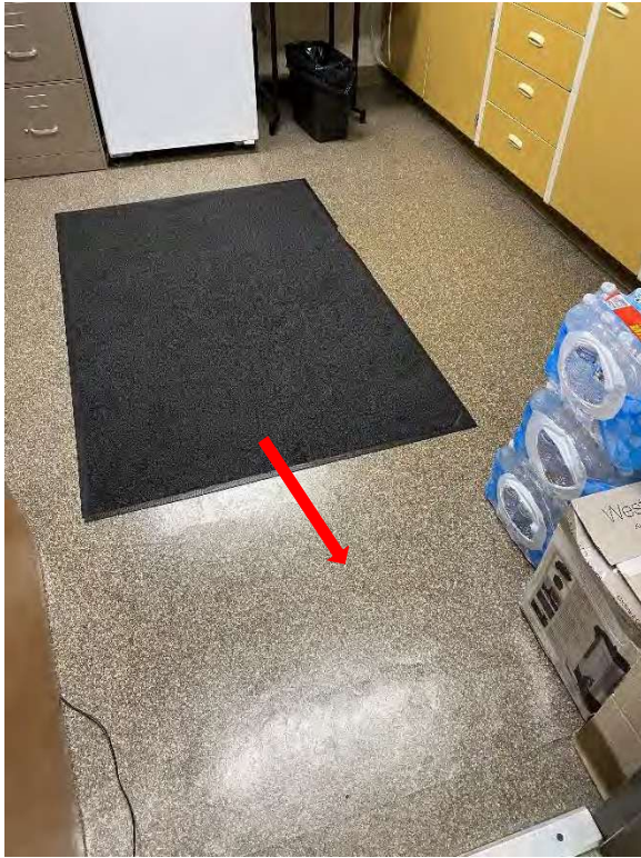
The gray sheet vinyl flooring and the yellow mastic used to attach it are asbestos-containing.
