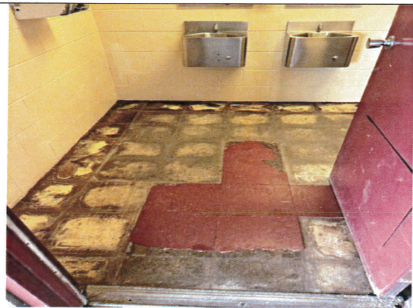
Men's Restroom with Wood ceiling, CMU Walls, and Red vinyl tile floor with black mastic. (Negative)
