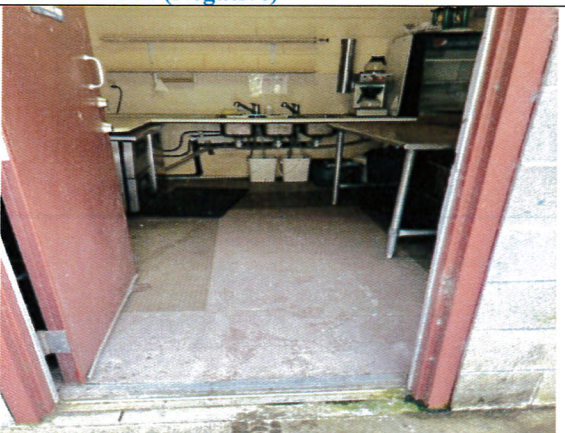
Concessions with Wood ceiling, CMU Walls, Sheetrock above grill and 2 types of vinyl tile floor. (Negative)
