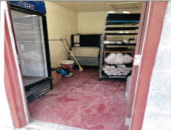
Storage with Wood ceiling, Cmu Walls, Red vinyl tile floor with black mastic and grey rubber cove base. (Negative)
