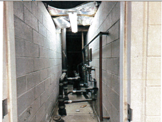
Pipes between walls in Locker Room. (Negative)
