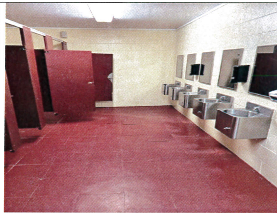
Women's Restrooms with Wood ceiling, Cmu Walls, and Red vinyl tile flooring. (Negative)
